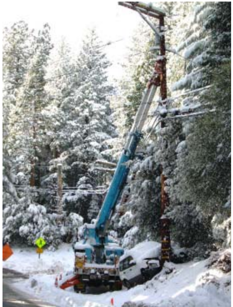
Power Pole Accident Scene.
